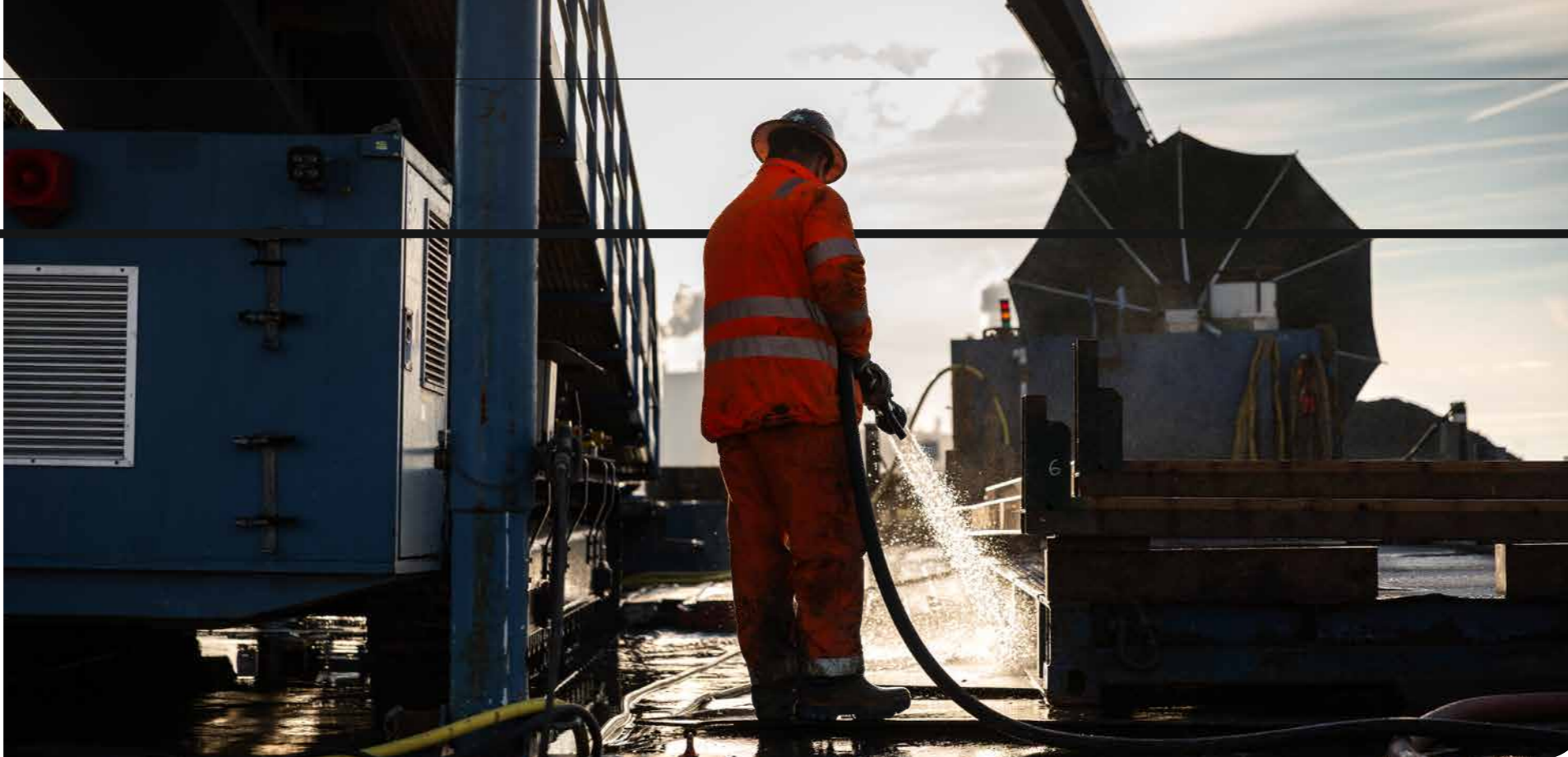
In Vlaardingen, Hanab is building the largest industrial waste heat capture facility in the world.
