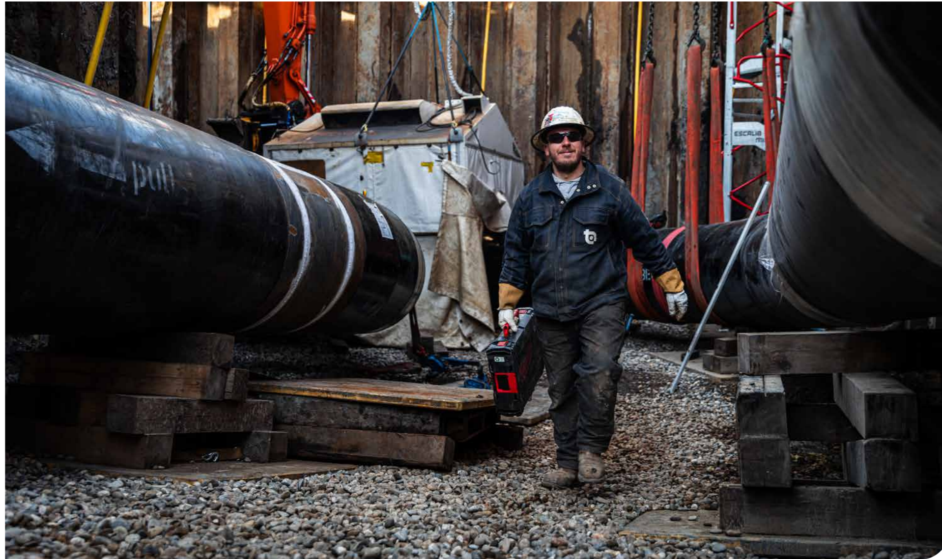
Over a distance of six kilometres, a new pipeline system is being installed in Vlaardingen for the supply and removal of industrial residual heat.
